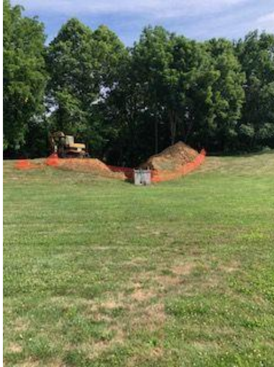
Photograph No. 1 – View across the SWM basin and the outlet structure at AOC. Photograph facing north
