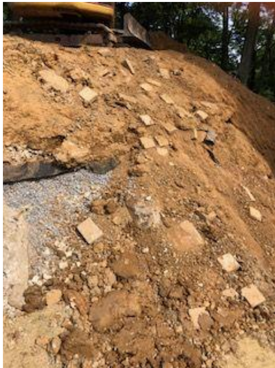
Photograph No. 14 – View of evidence of past repairs and materials used, along sidewall
