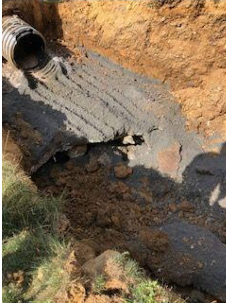
Photograph No. 5 – View behind outlet structure after pipe, anti-seep collar and portion of pad was removed. Note the void space and large rock beneath the edge of the concrete pad.
