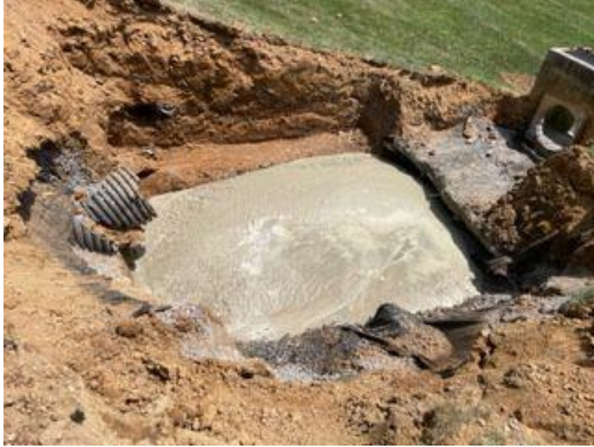
Photograph No. 9 – View of Photograph No. 8 area after backfilling with flowable fill.
