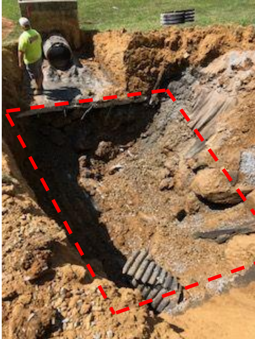
Photograph No. 8 – Additional view of first section of pipe removal and excavation of past repair and AOC areas. The area designated with RED represents a approximate picture of the area to be backfilled using low-strength cement flowable fill.
