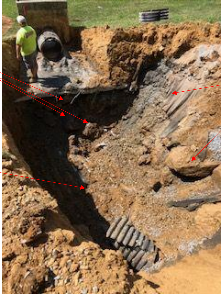
Photograph No. 7 – Additional view behind outlet structure. Note stacked rocks beneath past concrete pad repair and separate past sidewall repair (rock filter).
