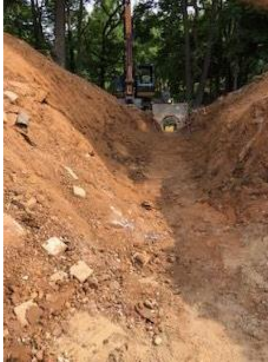
Photograph No. 15 – Remaining alignment after completion of existing pipe removal and subgrade preparation on July 9, 2024. Photo facing end wall.
