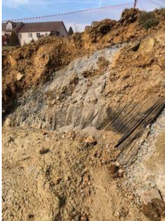
Photograph No. 13 – Flowable fill placement along western sidewall and past repair area, facing southwest.
